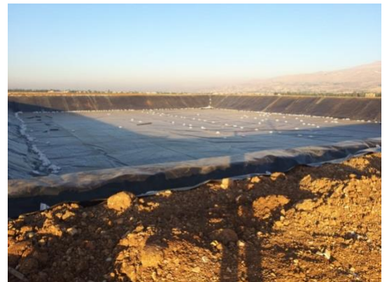
Pond completed with a geomembrane surface on the Gotextile and anchored at the crest of the slopes
